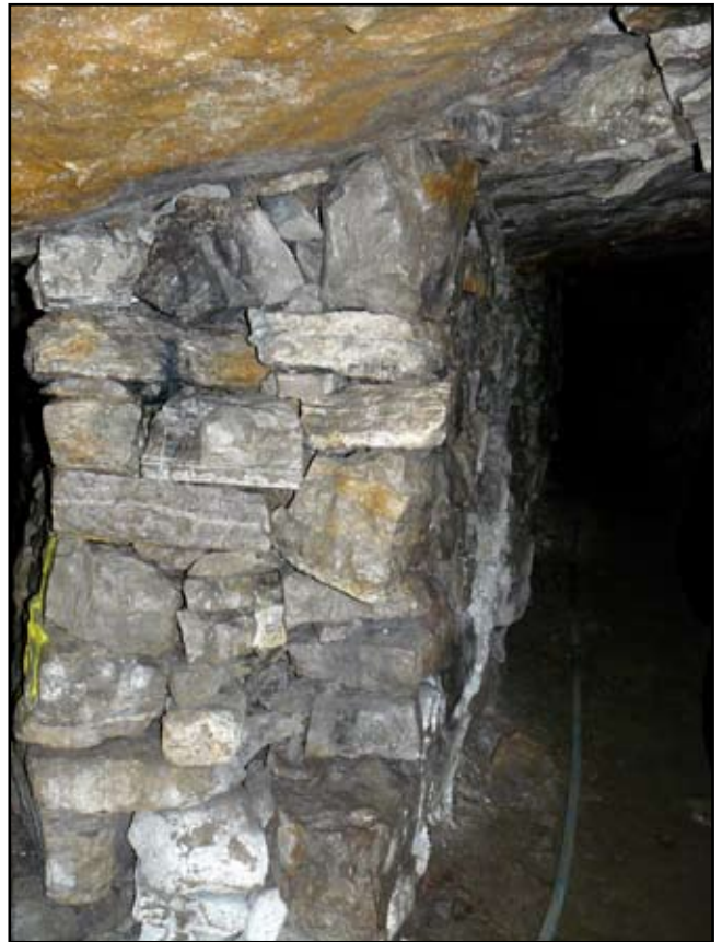
A roof support made of stacked limestone and chert waste in the Holme Bank mine.
